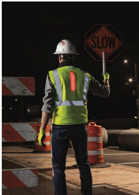
» Mobile maintenance staff should have lighted and reflective vests for proper visibility during roadside service.
